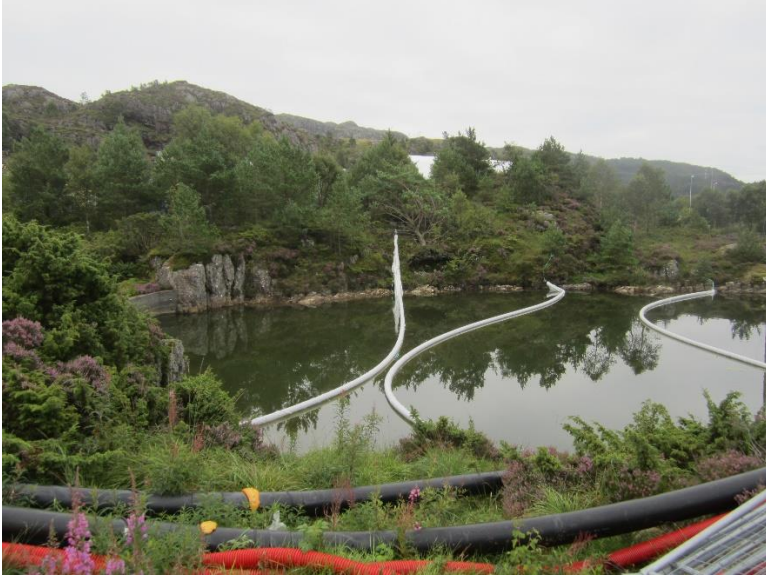
Figur 1 Utslipp rensed tunnelvann bak doble siltgardiner
